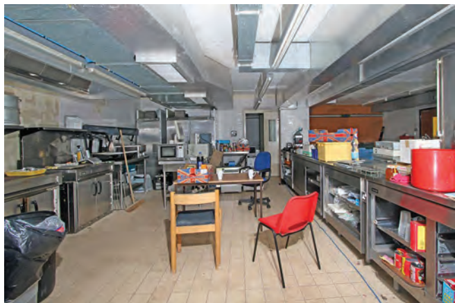
The high standard of fixtures and fittings in the well equipped kitchen is evident here. Everything is stainless steel including refrigerators and freezers which are seen in the background. The servery is to the right
